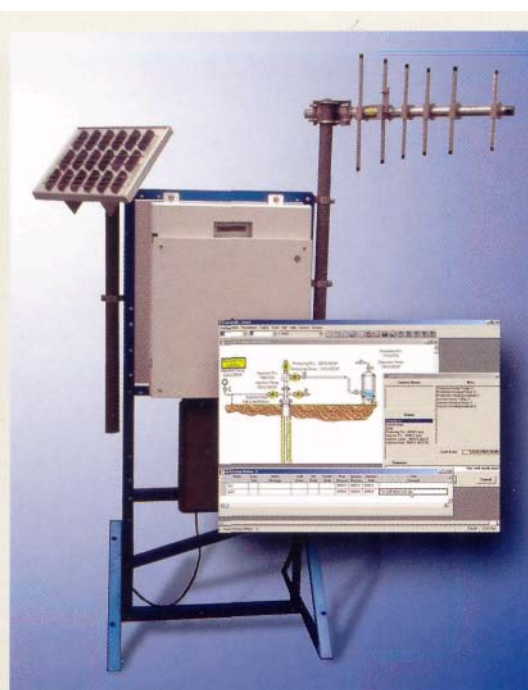
FIG. 10. Principal components of wellsite equipment and visual product of the Gas Lift Optimizer (GLO) controller.
